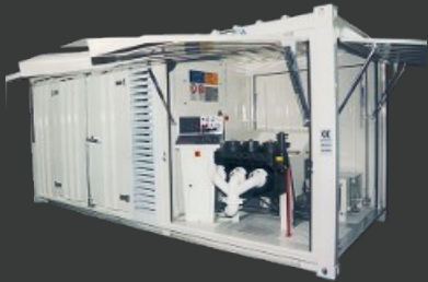
HIGH PRESSURE PUMPS
